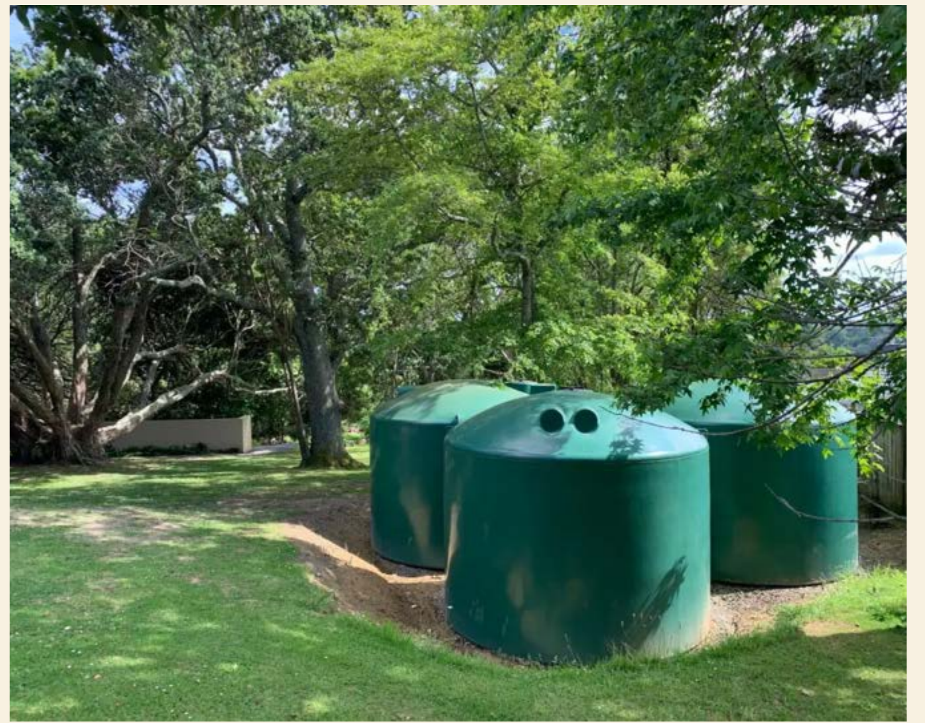
Rainwater storage tanks at the cemetery (photo: www.purewa.co.nz )
